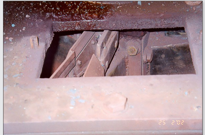
Figure 7. Vezin cutter aperture that is no longer radial due to poor maintenance.
