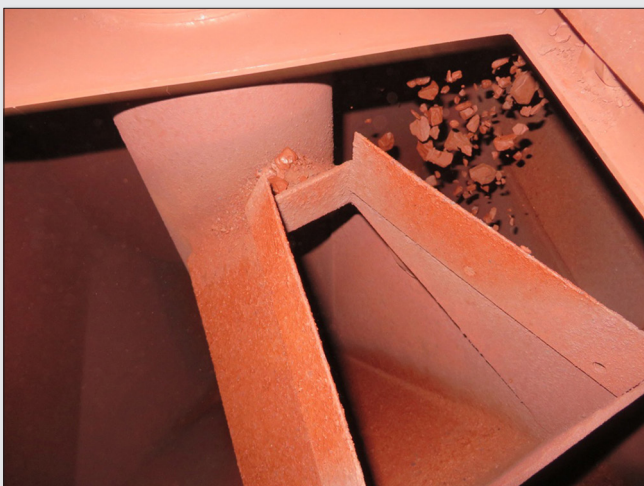
Figure 6. Example of a correctly designed radial Vezin cutter aperture just before interacting with the vertical falling stream of ore.
